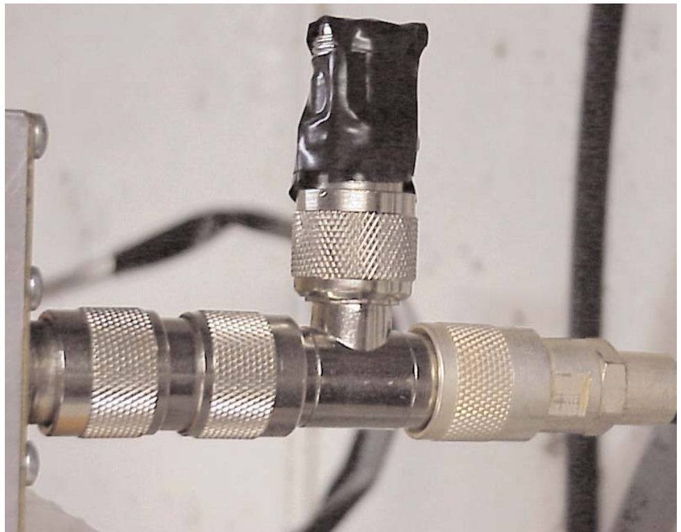
FIGURE 1: 70 cm 3-rd Harmonic Filter In-Line
